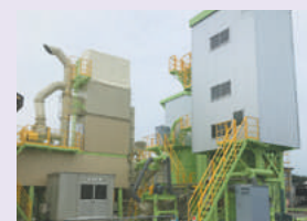
A plaster-based solidification material manufacturing facility A plant facility which manufactures gypsum hemihydrate from dried gypsum powder, which is blended with cement and lime to manufacture solidification material.
